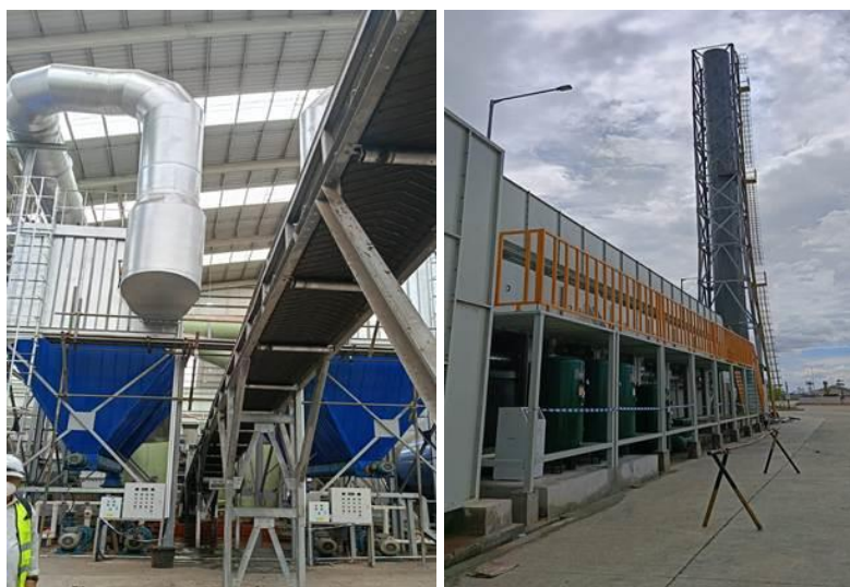
Gambar 4. Alat Pengendali Pencemaran Udara RDF Plant
